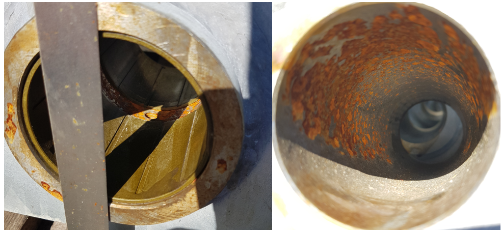
Illustration 2: Insufficient lubricant applied for basic corrosion protection
